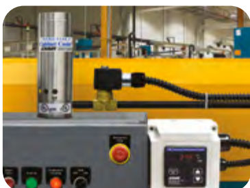
CABINET COOLER SYSTEM
