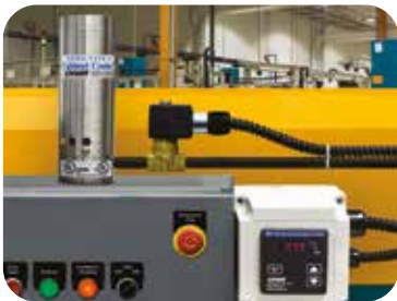
CABINET COOLER SYSTEM
